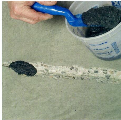
For larger spalls and cracks, Roadware 10 Minute Concrete Mender™ may be bucket mixed with silica sand and applied in bulk.
